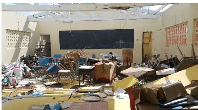
School damages in Barbuda (Photo credits: SPRINT-Lab, 2017)
